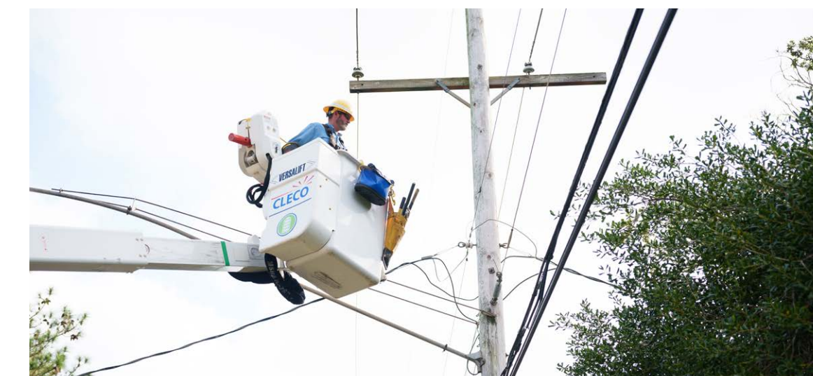
📷 Cleco electricity distribution network in Louisiana, US.
